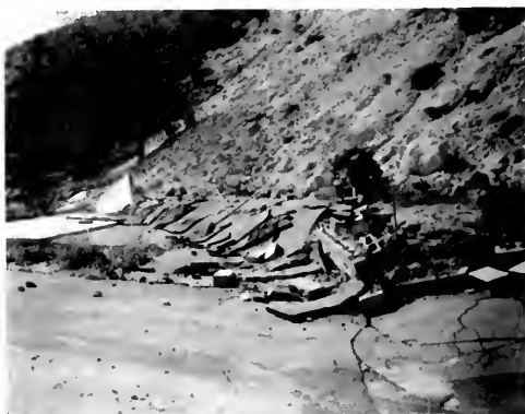
Photo 5. Deformed asphalt pavement and uplifted concrete slab along the 70 cm (2.3-foot) high scarp of the Tujunga fault segment in the Blue Star Trailer Park. Trench 8 (plate 4) was cut near shovel. Note also rockfall debris triggered by earthquake above scarp. Photo by James E. Kahle.
